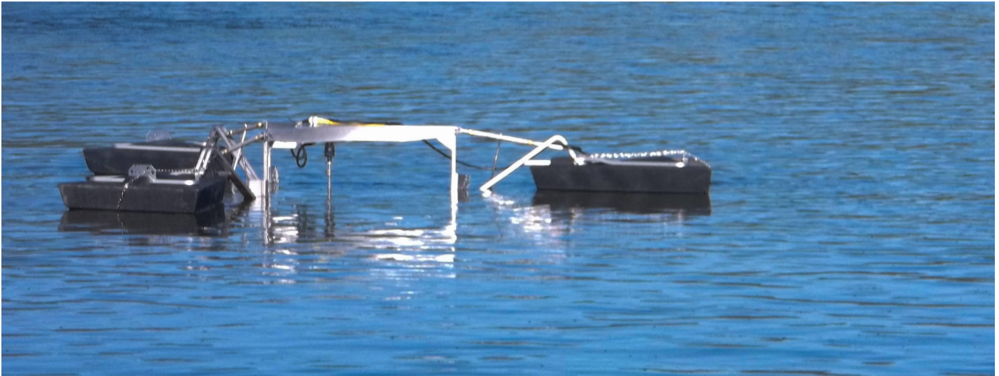
Floating wastewater mixers are a proven odor control strategy for many types of wastewater ponds and basins.
