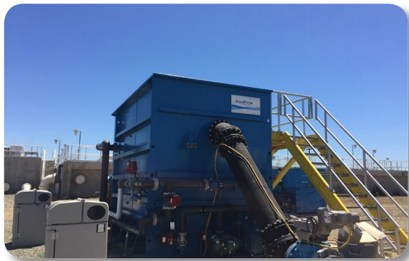
An AquaPrime® system operating at a municipality for primary treatment.
