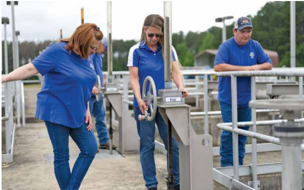
From left, Stacey Humphrey, Jennie Woods and Kenneth Moore waste sludge from the plant's sedimentation basin.
