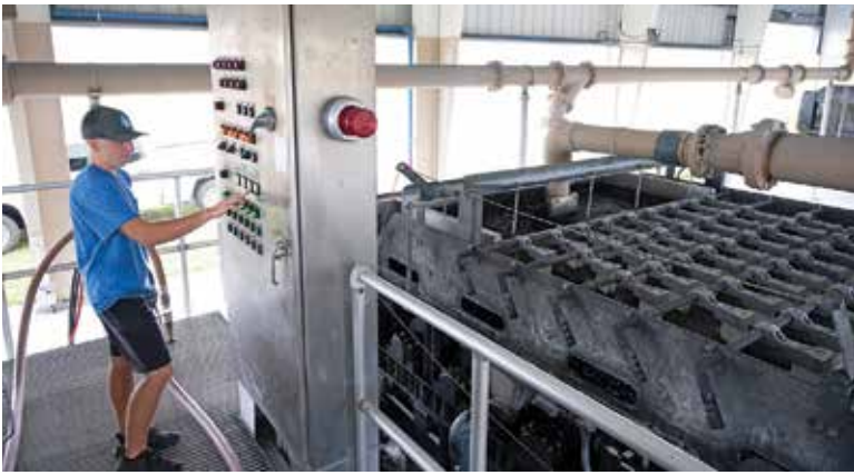
Biosolids are dewatered on belt presses (Alfa Laval) before landfilling. Jonathan Rivera, dewatering press operator, checks equipment operations.
