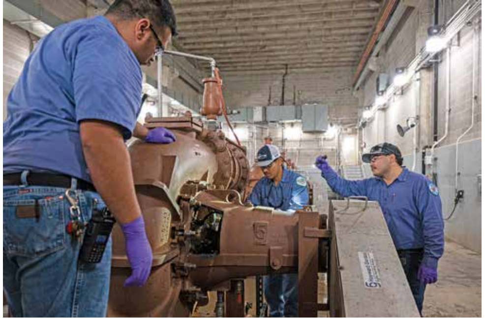
From left, Matthew Barber, operations and maintenance associate; Filiberto Castilleja, operations and maintenance supervisor; and Efrain Lopez, operations, conduct planned maintenance on equipment.
