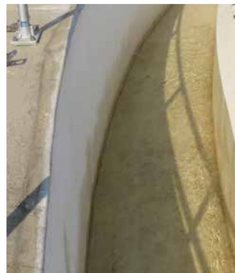
The launder area one year after the cover was installed, showing no algae and only a thin layer of biofilm.
