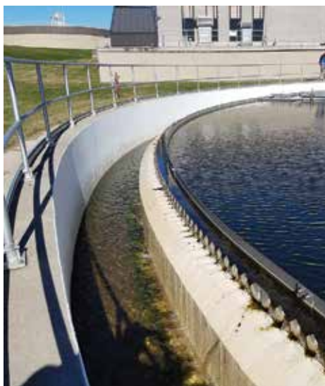
The launder and weir area before the cover installation with algae growth typical of conditions before the weekly cleanings.
