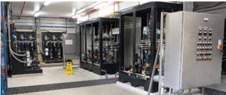
Controls for the Caterpillar and Cummins diesel generators that supply plant backup power.
