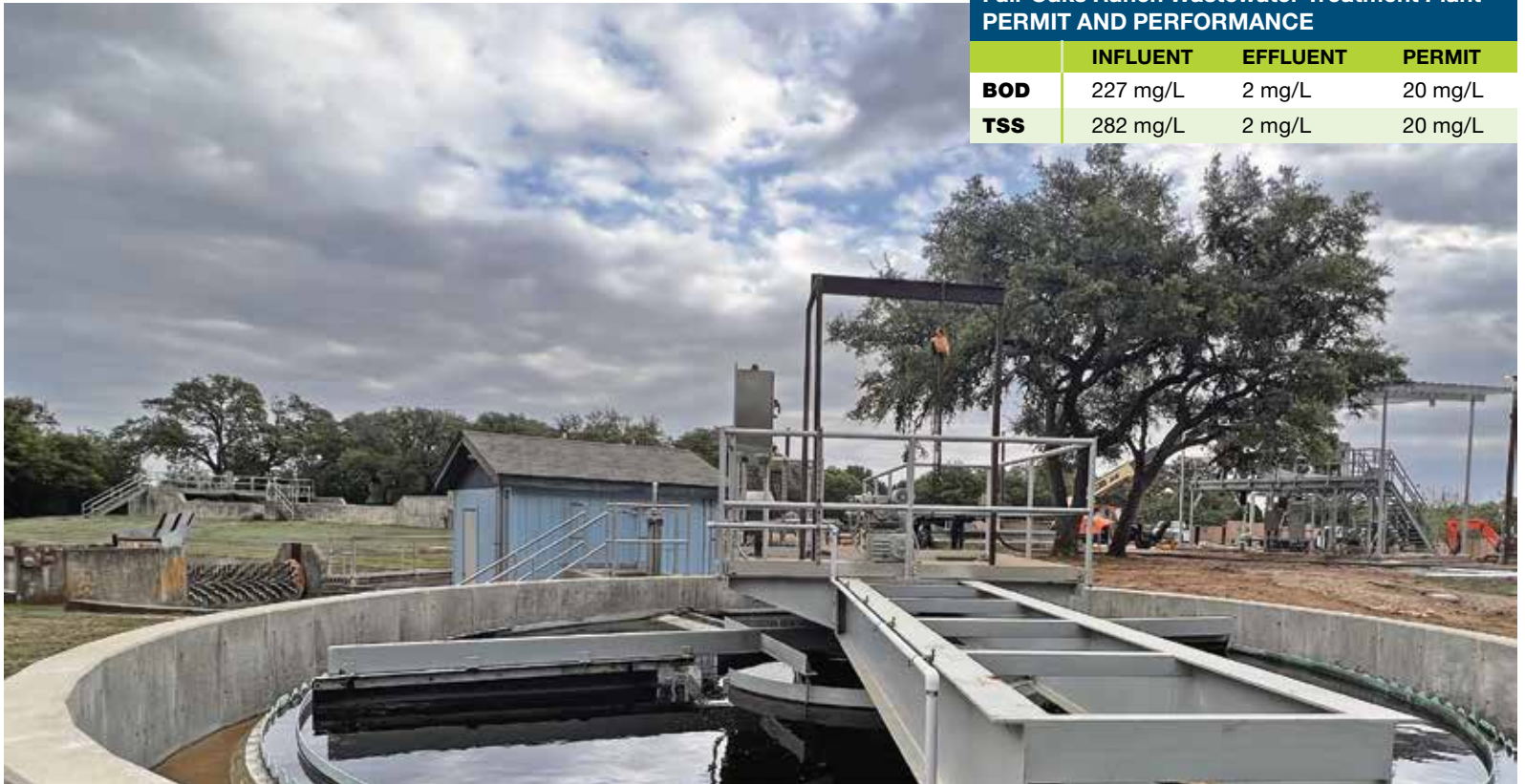
The Fair Oaks Ranch plant's record of excellence stems from process improvements and a dedicated staff (secondary clarifier from Envirodyne).
