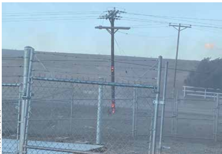
The site of the interconnect between the Louisville and Superior water systems, showing the swinging and flaming power pole nearby.
