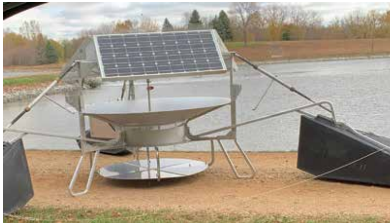
A SolarBee mixer sits on the shore before being floated onto the primary lagoon.
