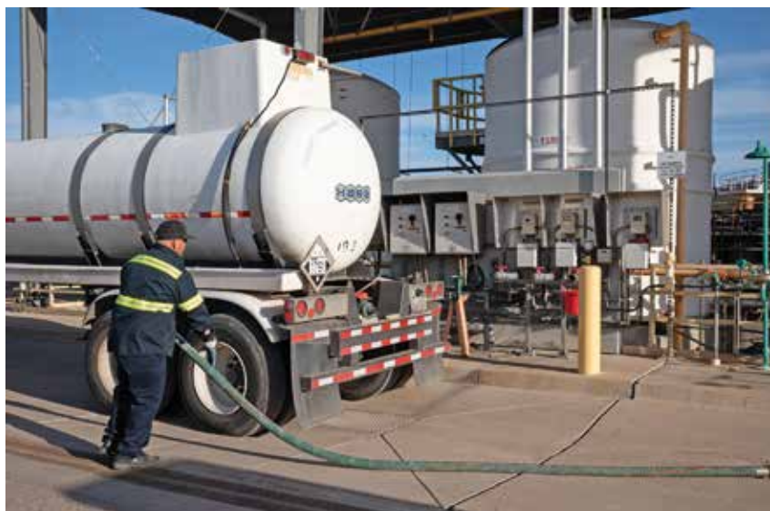
Frank Sanchez unloads sodium hypochlorite at the Tres Rios Water Reclamation Facility.
