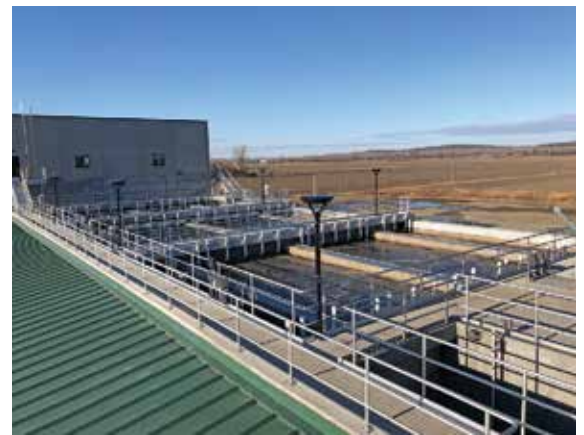
The process requires low long-term maintenance, and the installation provides flexibility to add another treatment train.
