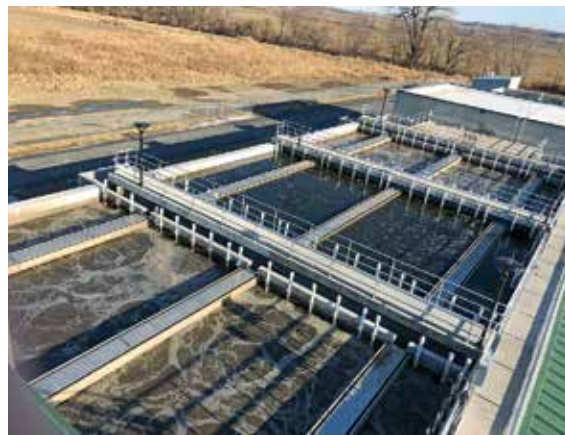
The AquaNereda process met a requirement for high treatment capacity on a compact footprint (Aqua-Aerobic).
