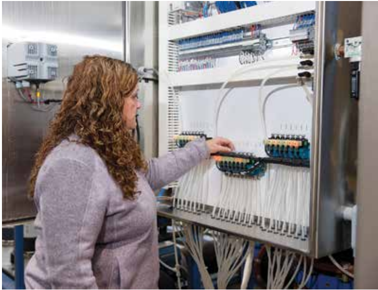
Grace Rixen’s key challenge in the past few years has been bringing new facilities online and training operators to run them at peak efficiency. She is shown testing the air valve for a membrane filtration system (Tonka Water).
